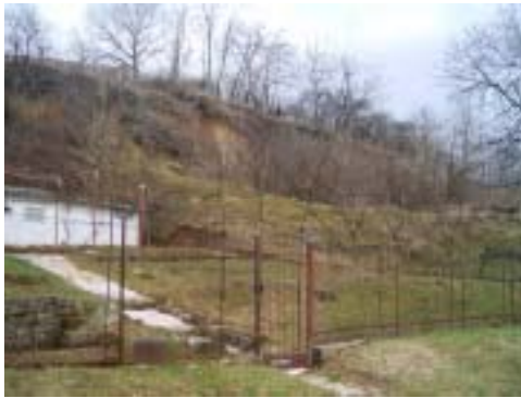
Zamca landslide base
