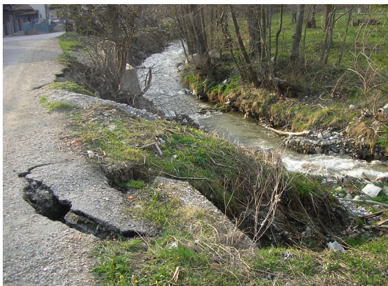
Fig. 1. Road degradation DC 51
