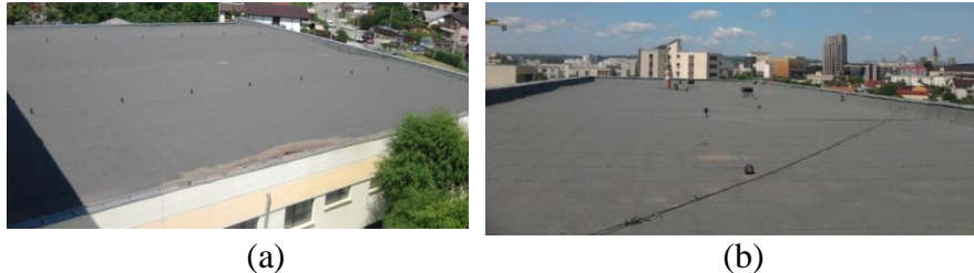
Fig. 1 –The roof surface of the (a) north building part, (b) south building part
