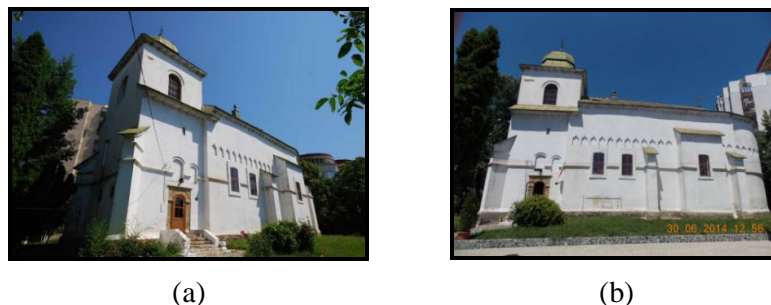
Fig. 1. The study building - “Vovidenia church” - perspective view of the south façade (a) south-west view and (b) south view
