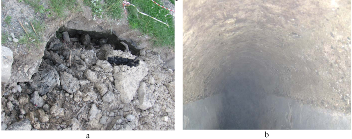
Fig. 2. Damage to the sewerage collectors domes visitors from concrete; a - collapse of the cover plate of a bell type sewerage; b - degradation of concrete on the underside of the cover plate to an ovoid type sewerage.
