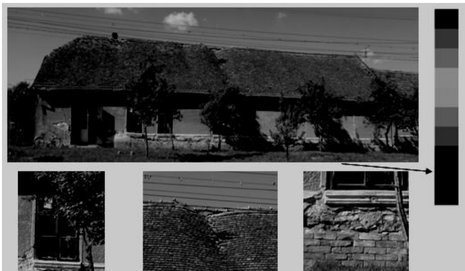
Fig.4. House – type 3 Old house of unfired bricks, damaged plaster, PVC window, old rooftop
