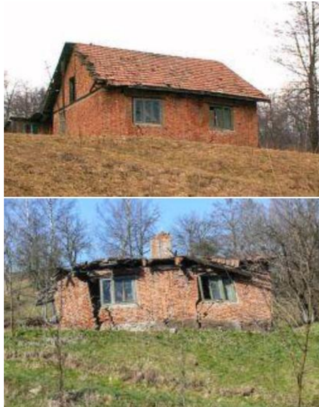
Figure 1. The negative effects of subsidence. Building existing in the influence area of the layer 3 operation, Block III – Comparison between February 2008 and April 2015, Petrila. [2].
