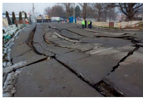
Fig. 6 Secondary displacements around the cone, Street M. Eminescu
