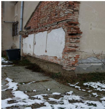
Fig.1 Slope Deterioration - Right Side Facade
