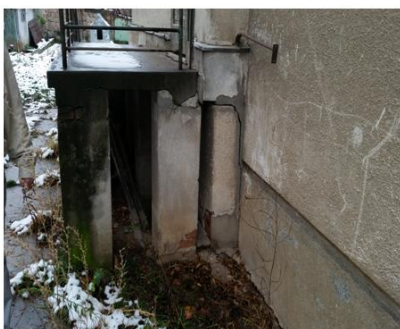
Fig.3 Cracks in the left side facade
