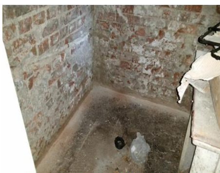
Fig.7 Lime deposits on mortar
