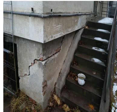
Fig.2 Cracks in Rear Facade
