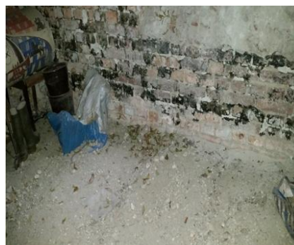
Fig.8 Ineffective intervention by application of a molten bitumen layer
