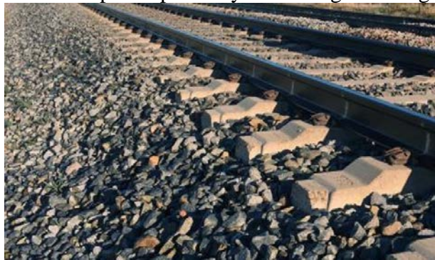
Fig. 2 Broken Stone Prism
