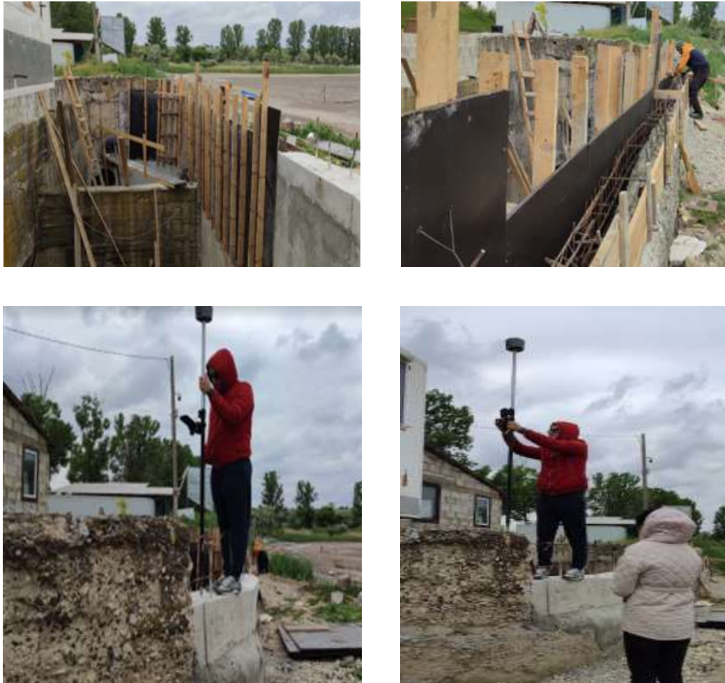
Figure 2. Geodetic works for the rehabilitation of the large water spillway structure, including the surveying and verification of characteristic points
